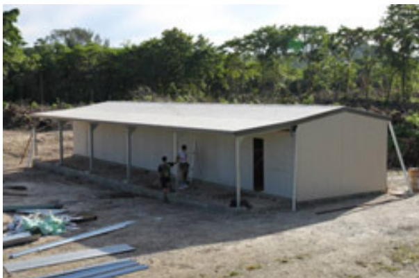
The framing, cladding and plumbing was complete when this photo was taken
